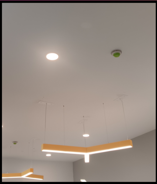
Photo of new light fixtures in the community room.
